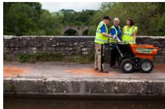
Towpath repairs on the Brynlich aqueduct on the Monmouth & Brecon Canal (Canal & River Trust)
